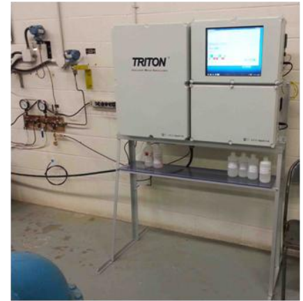
A TRITON unit in operation at London's Pond Mills Pumping Station.
